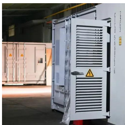
Pilot 120kWh battery energy storage system ...
