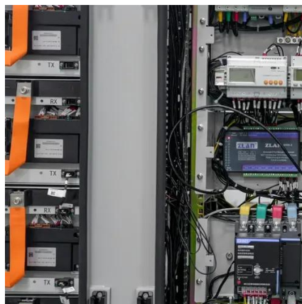
Commercial ESS 150kW/300kWh - EnSmart ...
