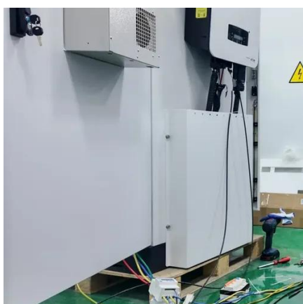
Battery Energy Storage Systems
