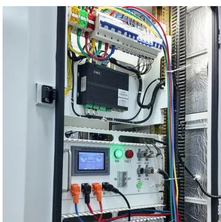
20kW energy storage cabinet
