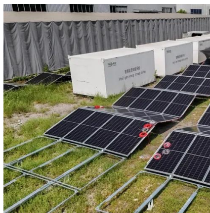
Solar panels board & power bank
