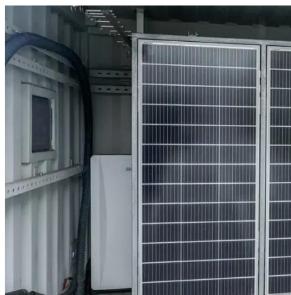
Netsure731 48V 30KW Network Server Rack Cabinet R48 ...
