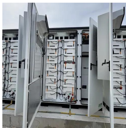
30Kwh Rack Mount Lithium Battery Storage Cabinet
