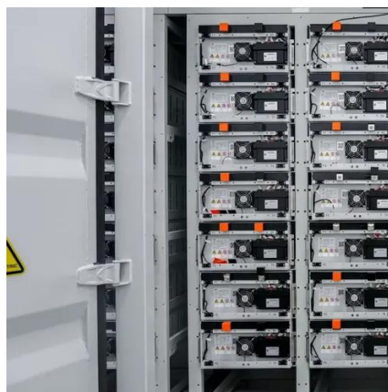
monrovia heavy industry energy storage cabinet
