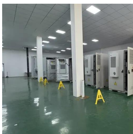
Deye GE-FL60 cabinets, 60kwh battery bank with ...
