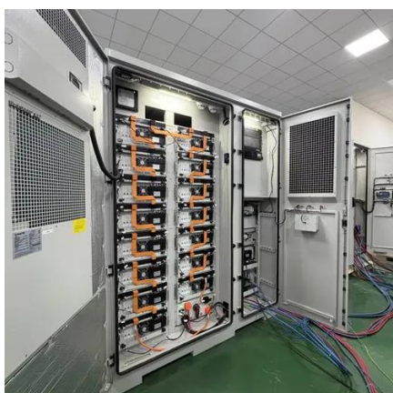
30KW/60KWh C&I All-in-One ESS ...
