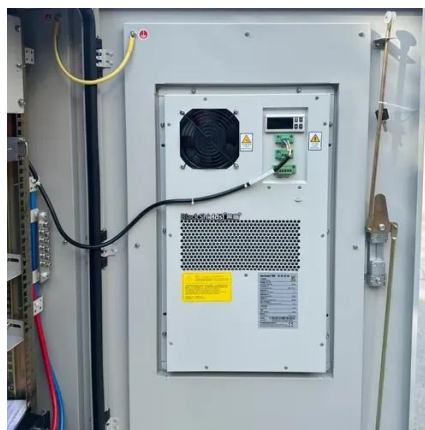
Deye GE-FL60 cabinets, 60kwh battery bank with IP65 ...
