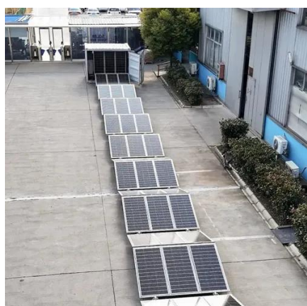
PV Grid-Connected Cabinet , Low Voltage Distribution Board , IPKIS
