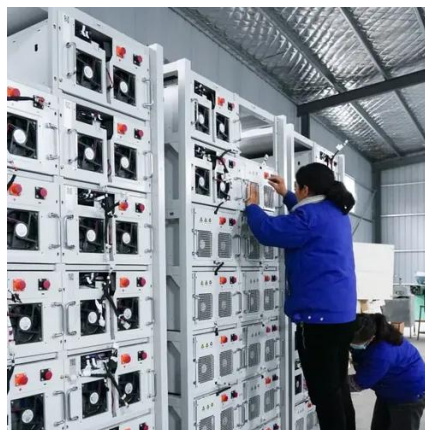
BESS 1MW 3.2MWh AC 480V Three Phase ...
