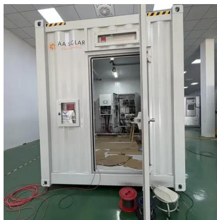
Energy storage container, BESS container
