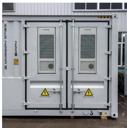
75kw dc energy storage unit
