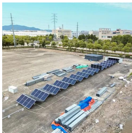
Solar lithium battery storage system installed in Lebanon! 40kWh ...
