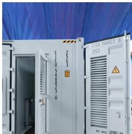
STORAGE CABINET , Solar Power Solutions
