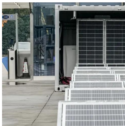
Battery energy storage system (BESS) container. ...
