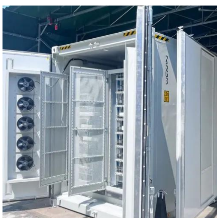
GSL ENERGY Commercial and Industrial Storage ...
