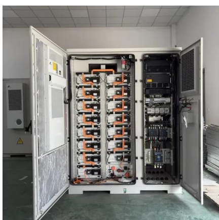
Photovoltaic Grid Cabinet
