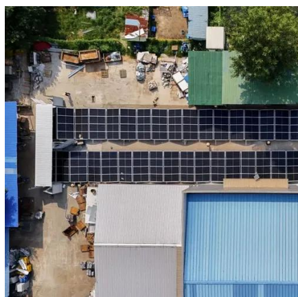
SHANGHAI ELECNOVA ENERGY STORAGE ...
