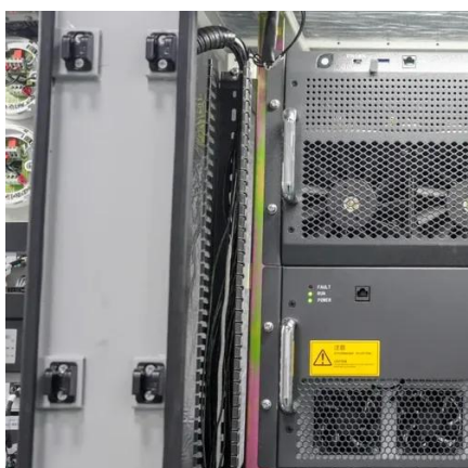
Outdoor Cabinet , SWA Energy LiFePO4 Battery Storage Systems
