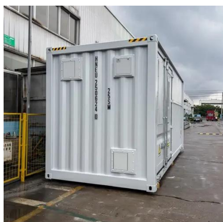
Single Phase Primary Cabinets, Two Phase Primary Cabinets, Three Phase
