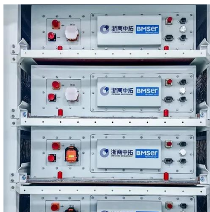
Huawei Luna 2000 , Huawei Battery System ...
