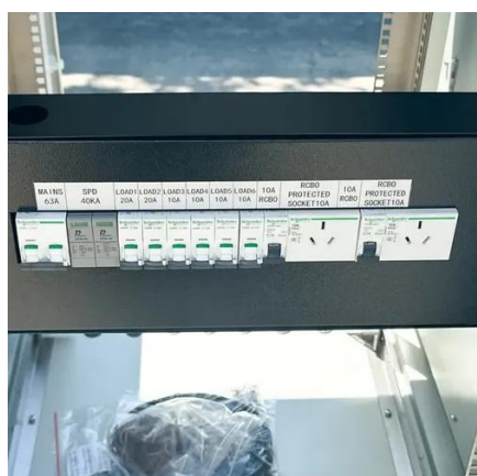
How To Choose The Right Server Rack Battery
