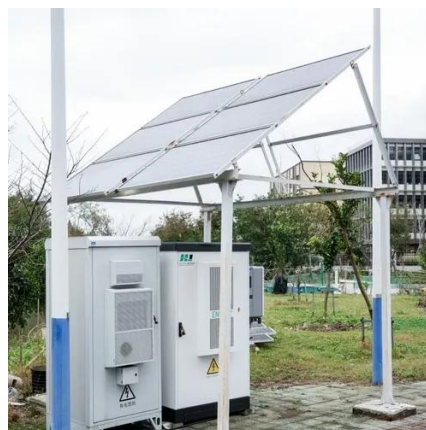
150kw energy storage cabinet
