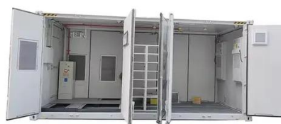
1075KW HH ESS
