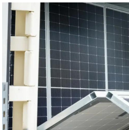
Photovoltaic energy storage power station Khartoum
