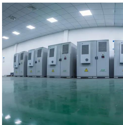
Commercial ESS, 100KW 215KWH Off-Grid System
