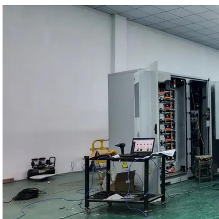
Ljubljana Power Exchange , C& I Energy Storage System
