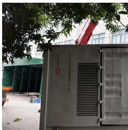
Lusaka Green Container Energy Storage Enterprise
