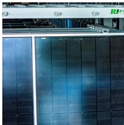
Inside a 1 MWh Energy Storage System Heading ...
