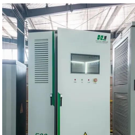
Commercial & Industrial Storage BESS System ...
