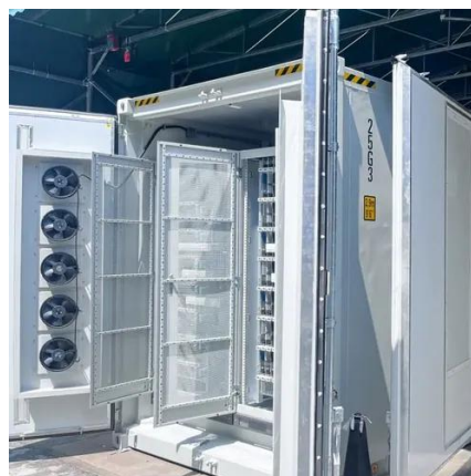
Energy storage container, BESS container
