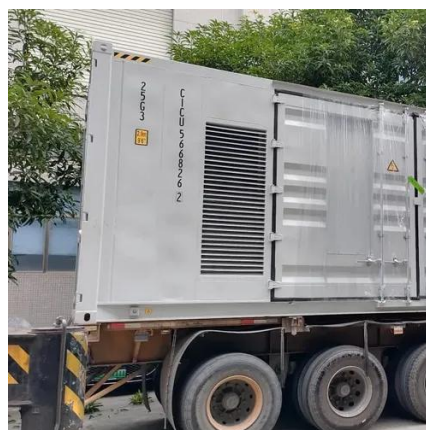
Utility-scale battery energy storage system (BESS)
