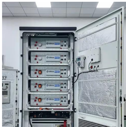
Micronesia battery storage cabinet
