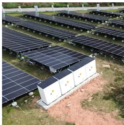
Mobile Solar Containers , Green City Times
