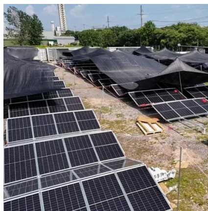
Bluesun 600kWh energy storage system in #myanmar
