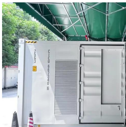
Micro Grid Energy Storage. Energy Cabinet. Container Energy Storage
