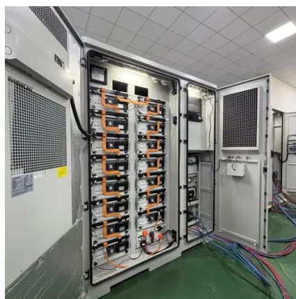
Dawnice 200kWh Battery Storage Systems
