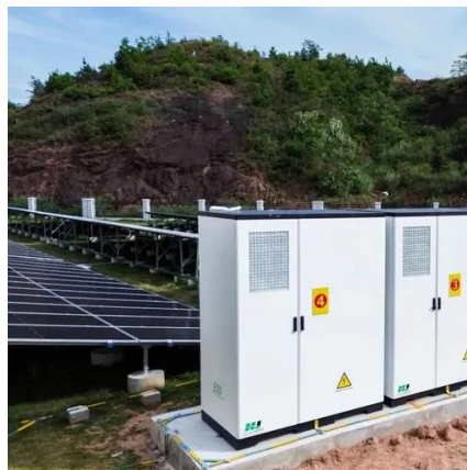
Substation explosion-proof lead-acid battery cabinet
