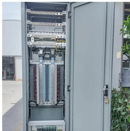
China Telecom Cabinet, Telecom Cabinet ...
