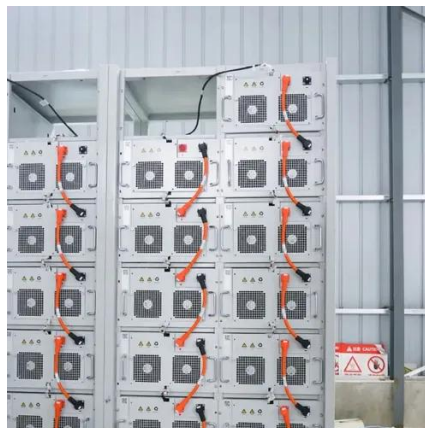
Container Bess Solar Battery Energy Storage ...
