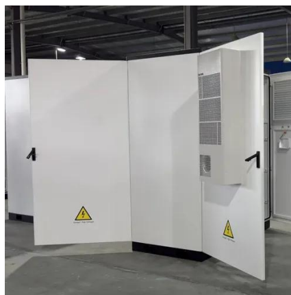
Outdoor power cabinet
