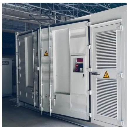
Outdoor Communication Cabinets and Power ...
