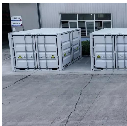
100 kWh Battery Commercial Energy Storage
