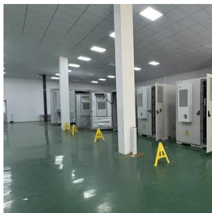
Tirana photovoltaic energy storage battery , C& I Energy Storage ...
