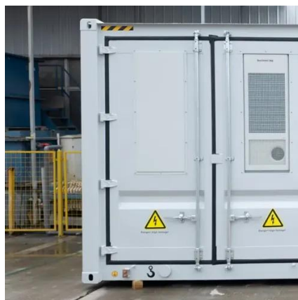
Energy storage battery cabinet Estonia
