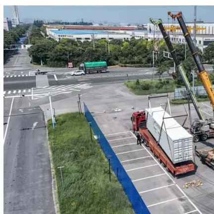
Energy storage battery cabinet Estonia
